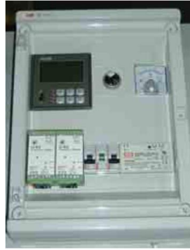
Figure 2.3 Electrical power measuring and recording device
