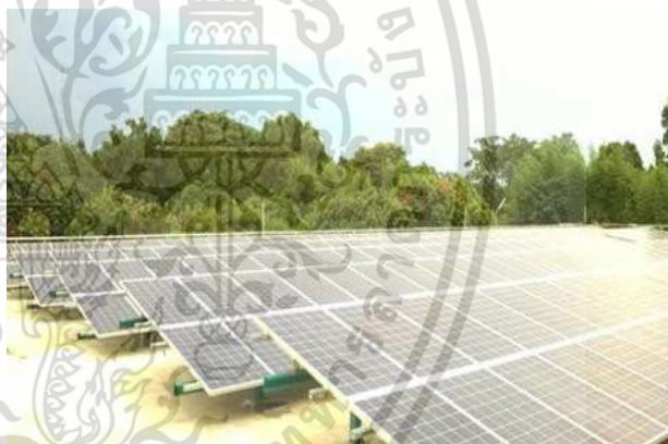
Fig.2 PV system installed in Kampong Thom Province, Cambodia
