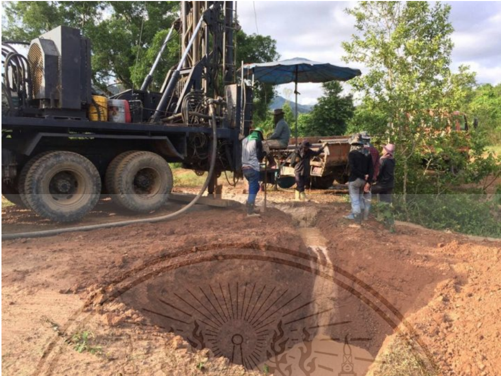
Figure 1.3: Groundwater wells in Kuiburi to solve the water shortage problem [16]
