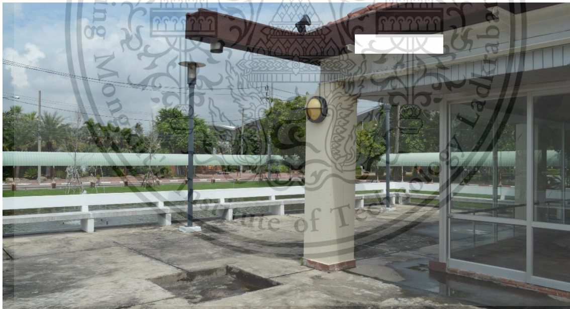
Fig. 37 Rain water drain system in cafetorium (Photo by author)
