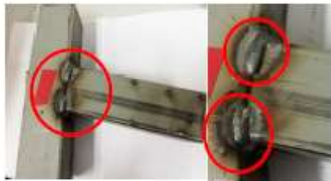
Fig. 18 Deformation Behavior for Corner welded group 2
