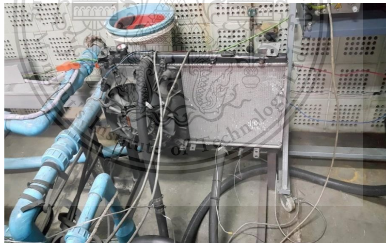
Figure 3.5 External Radiator System
