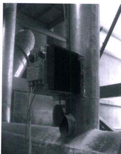
Figure 3.4 Installation of a diode-array in-line NIR spectrometer (DA7300, Perten, Sweden)
