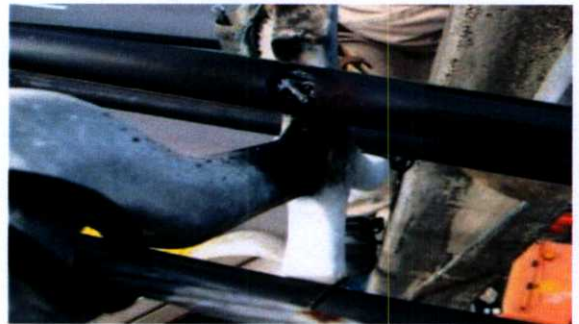
Fig. 1. a) SAC construction b) SAC for distribution system. c) Surface tracking problem of the installed SAC
