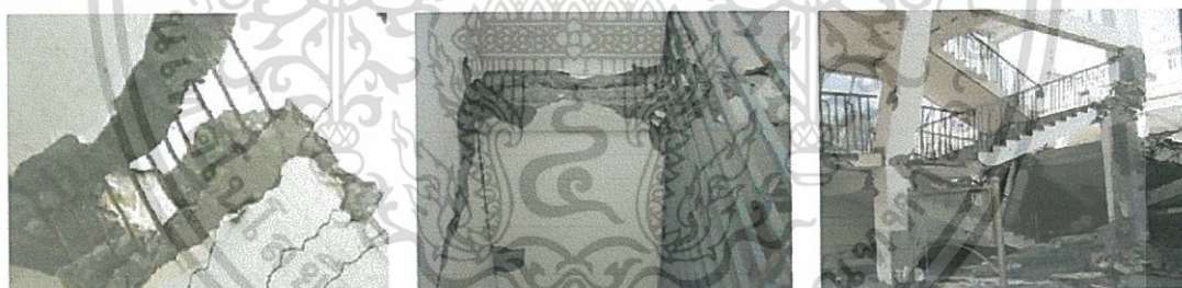
(a) Fractures of staircase slabs (b) Damages of landing beams (c) Damages of frame columns
