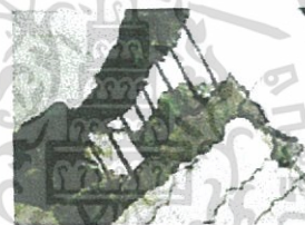
(a) Fractures of staircase slabs
