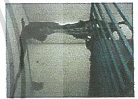
(b) Damages of landing beams
