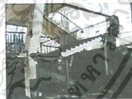
(c) Damages of frame columns
