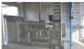
Figure 16. a 130 kW methane-gas generator used in this test
