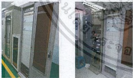
Fig. 9. (Left) Teleprotection cabinet installed at ABCD and (Right) Teleprotection cabinet installed at EGAT-RY1 substation
