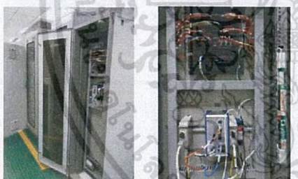
Fig. 10 RTU cabinet installed at ABCD Power Plant
