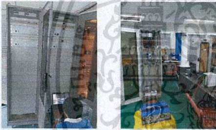
Fig. 8. (Left) FAT test of the Teleprotection cabinets and (Right) FAT test of an RTU cabinet
