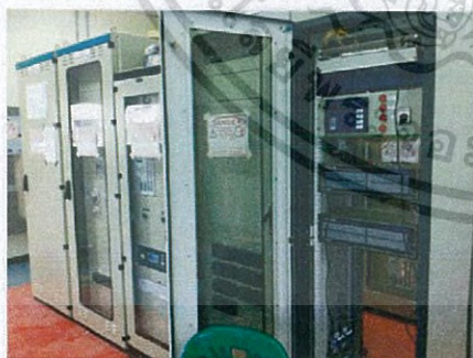
Figure 6. Logic processor hardware in control room.
