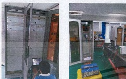
Fig. 8 (Left) FAT test of the Teleprotection cabinets and (Right) FAT test of an RTU cabinet
