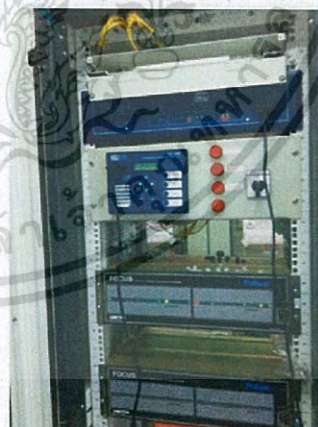
Figure 7. Logic processor hardware in control room.
