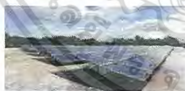
Fig. 4 The 126 kW p PV system
