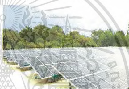
Fig.2 PV system installed in Kampong Thom Province, Cambodia
