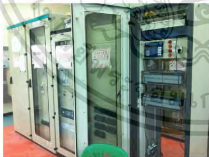
Figure 6. Logic processor hardware in control room.
