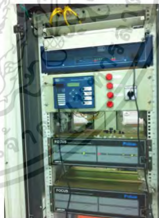
Figure 7. Logic processor hardware in control room.
