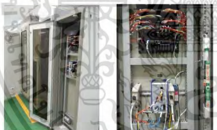
Fig. 10 RTU cabinet installed at ABCD Power Plant
