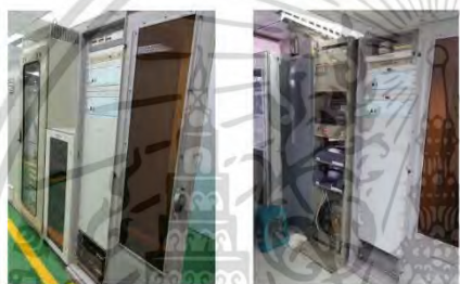
Fig. 9 (Left) Teleprotection cabinet installed at ABCD and (Right) Teleprotection cabinet installed at EGAT-RY1 substation
