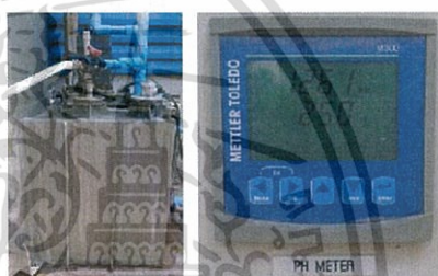
Fig. 19 Installation of the pH meter in the scrubber.
