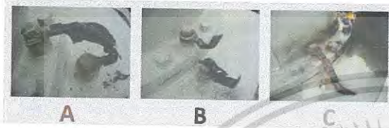
Fig.6 Burned ground wires during a commissioning test
