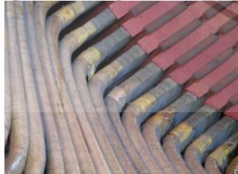
Figure 4. The dust found on the surface of stator winding insulation
