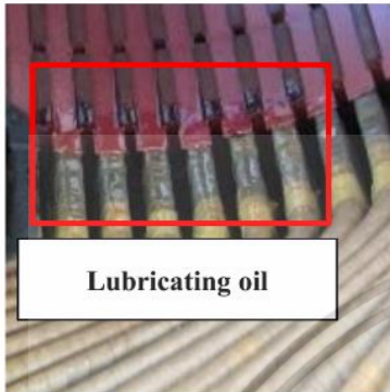
Figure 11. Lubricating oil applied on the surface of stator winding
