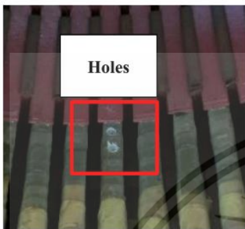
Figure 15. two holes damaged on the surface of stator winding insulation
