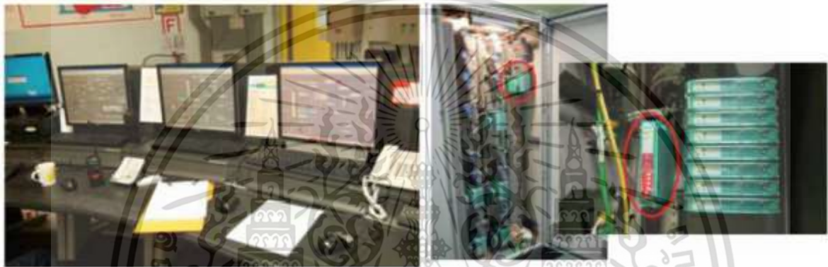
(b) In the control room
