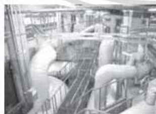
Centralized management of lifelines [Joint utility tunnels]
