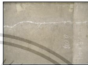
(c) Crack at concrete deck
