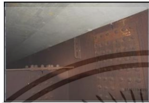
(b) Corrosion of steel box girder
