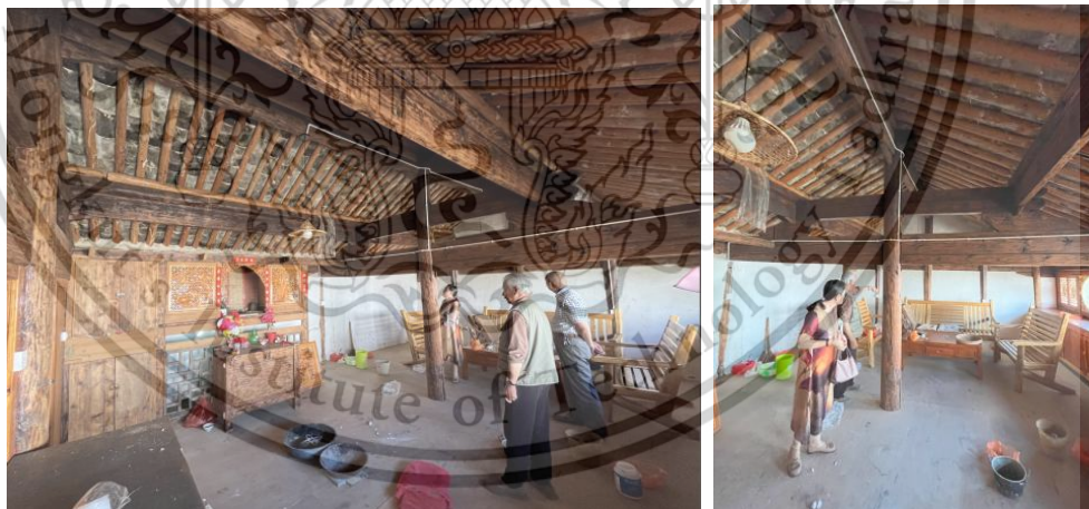
Figure 0.9 On the second floor, one wall was removed to make the space open and bright, and only one room was kept, which is now a storage room. In the picture, there is a shrine on the left and a desk on the right, where the old man of the family used to write with a brush. The beams and pillars of the house have been polished and are not so old.
