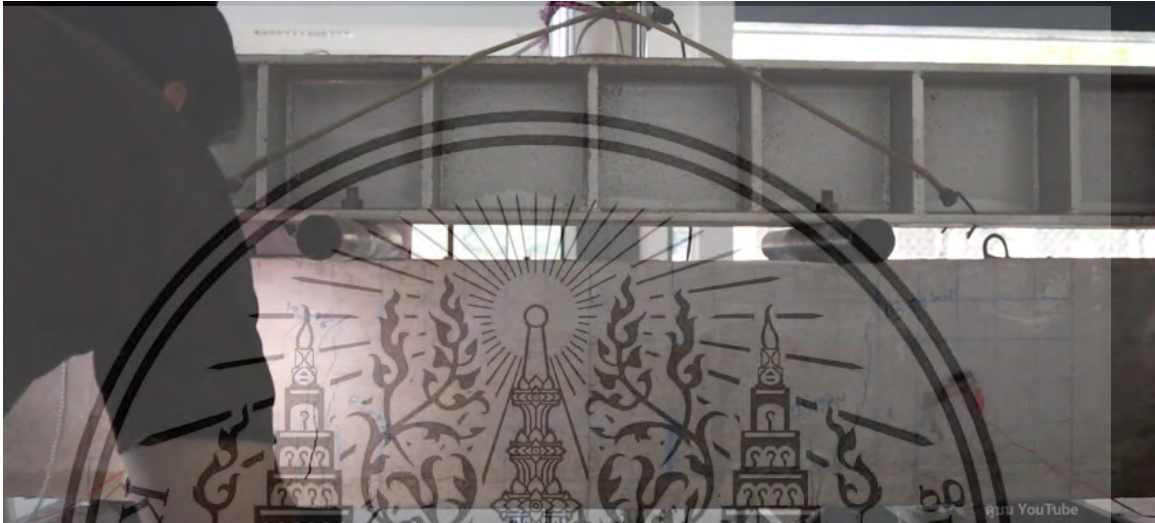
Figure 51 : Record and draw the cracking of the beam.
