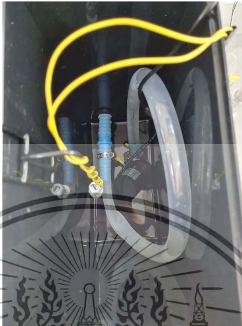
Figure 3. 17 Inside the water tank with water sensor and pump
