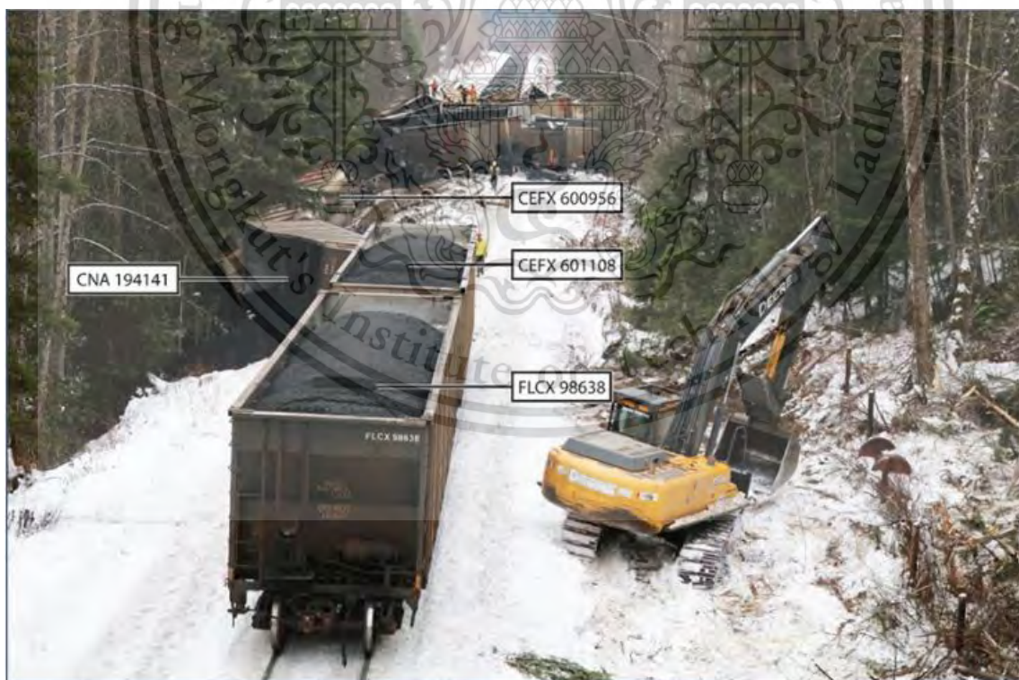
Figure 2.5 Eastward view of the derailed cars (Source: Interior News, with TSB annotations)
