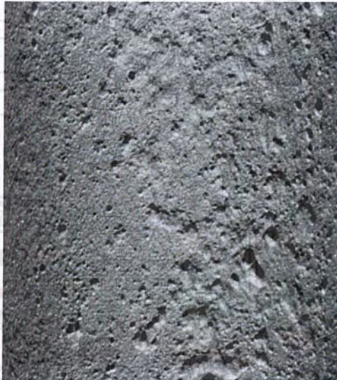
Figure 2.3 Oxygen pitting of economizer feed water inlet
