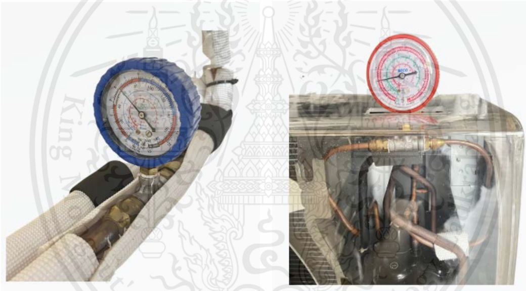
Figure 4.2 Pressure gauge evaporator and condenser at inside
