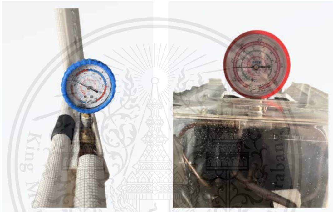
Figure 4.1 Pressure gauge evaporator and condenser at outside
