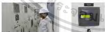
Fig. 19. Shows the results of the installation of the 5 th filter at transformer 1
