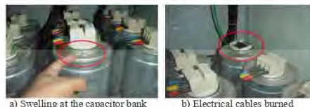
Fig. 15. Damage of the 7% Detune filter (12 x 50kVAR, 400V)
