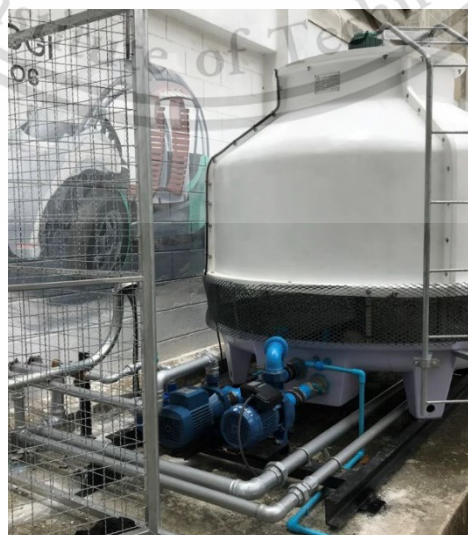
Figure 3-6 Actual photo of water-cooling tower
