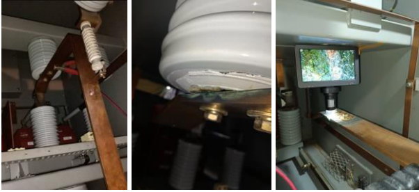
Fig. 5. the PD source inside the exciter transformer
