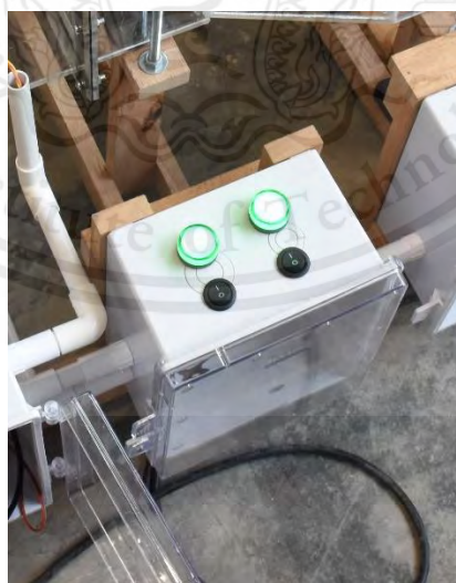
Figure 3.63 Low voltage box top view.
