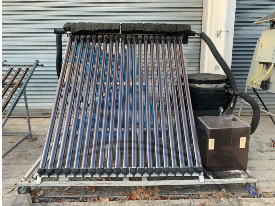
Figure 3.2: Evacuated tube solar collector in the experiment
