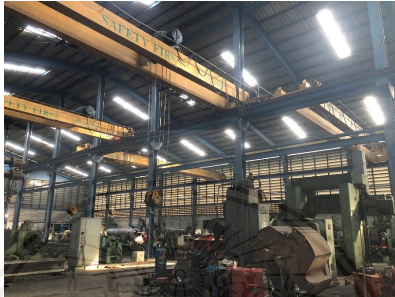
Figure 6.8: Crane in factory of Sahamit Metal Industry Company
