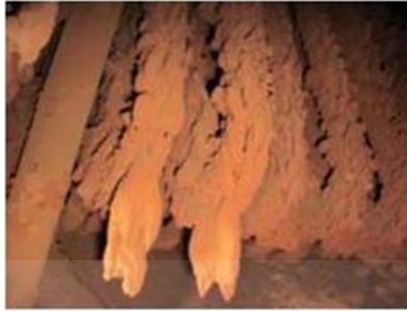
Figure 1.1 Superheater tubes in a coal fired boiler.
