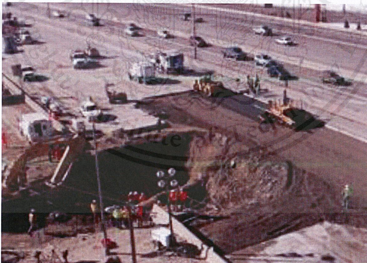
Figure 2.4. 66-in water main ruptures as a result of hydraulic initiated by a pump failure (Leslie, 2008).
