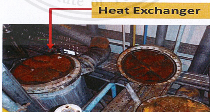
Figure 1.1 Rust clogged at the heat exchanger in the chilled water system (Momentive Performance Materials (Thailand) Limited. 2019)
