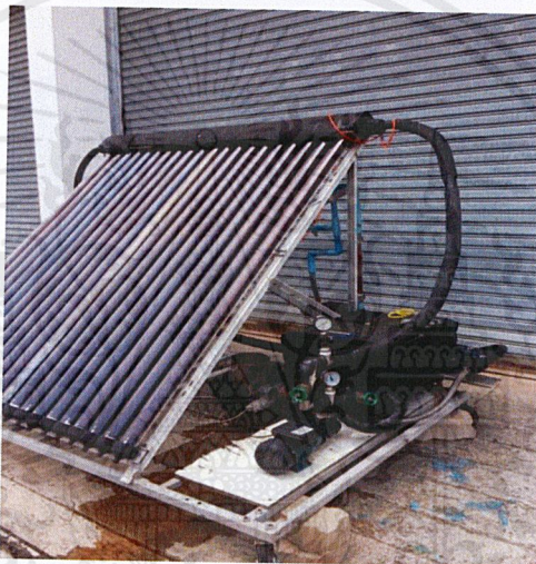
Figure 10: the system is covered by aeroflex-standard insulator
