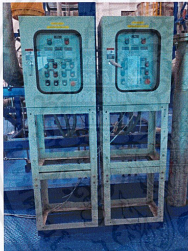
(c) ตู้ Junction Box PLANT-C
