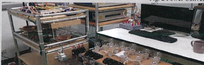
Fig. 3 Battery Energy Storage System and Demonstrated Microgrid
