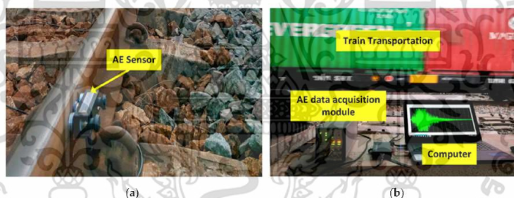
Figure 15. Onsite experiment on steel rail using the AE scheme: (a) installation of the AE sensor on the steel rail; (b) AE signal data of the steel rail under a load.
