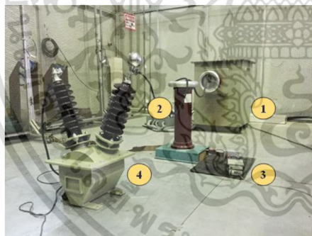
Fig. 6. Experimental test set up of the partial discharge test with the PT.
