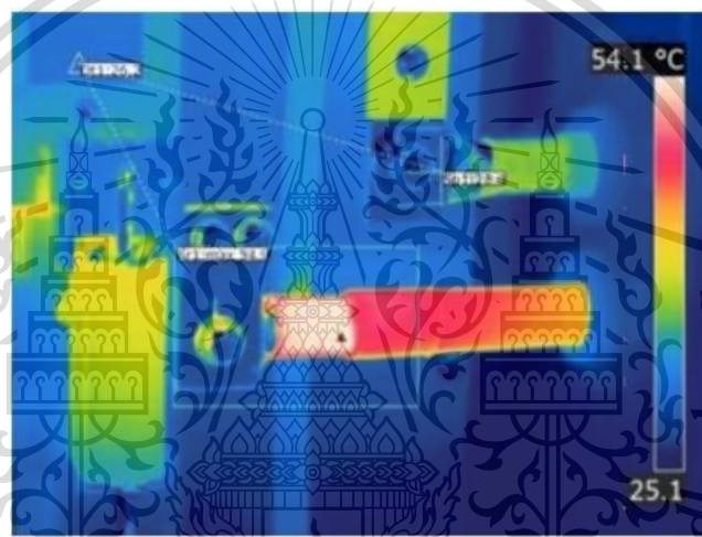
รูป 2.35 DC Combiner box overheated
