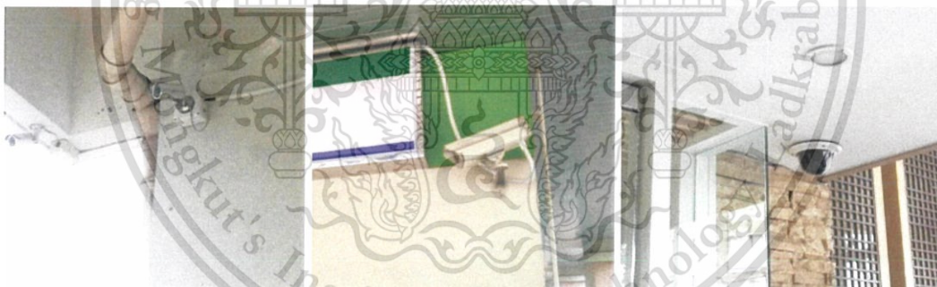
Figure 6.6 CCTVs camera of the condominiums
