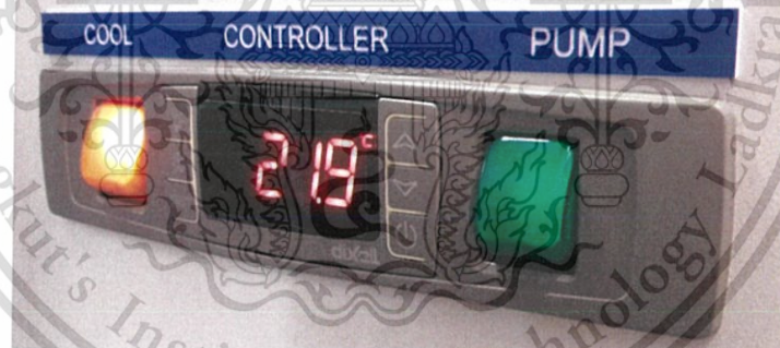
Figure 3.5 The panel of the cooling system.
