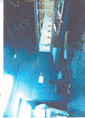
Control room is on the 2nd floor. This room have to point with dark color and dimmer light.
