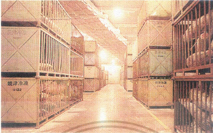
-55°C cold storage room
