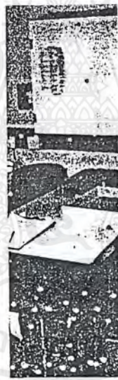
Fume cupboard controls
