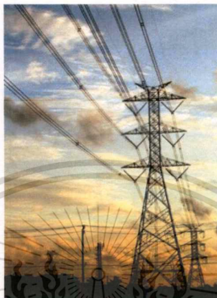
Figure 2.22: High voltage electricity post
