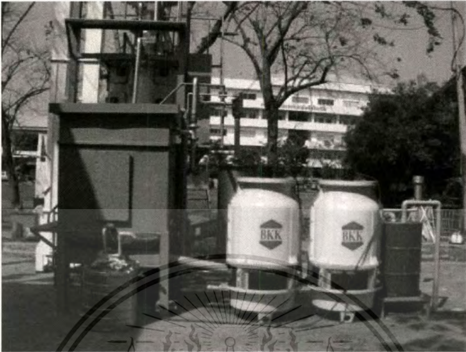
Fig. c.4. The cooling tower (yellow).
