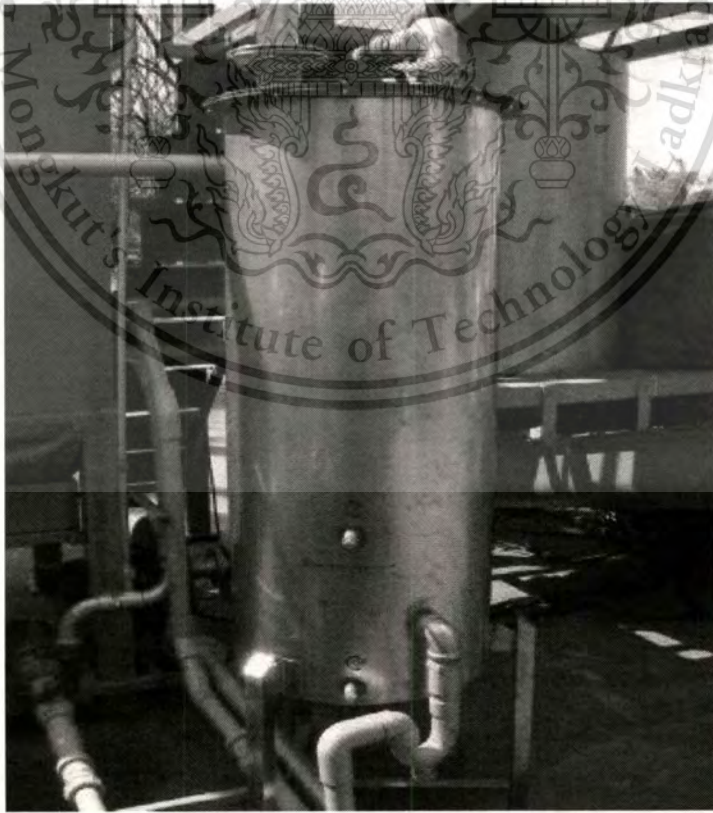
Fig. c.13. The gas treatment unit.
