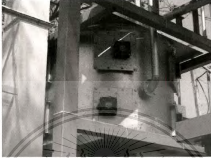
Fig. 4.2. A snapshot of the heating system of the carbonization reactor.
