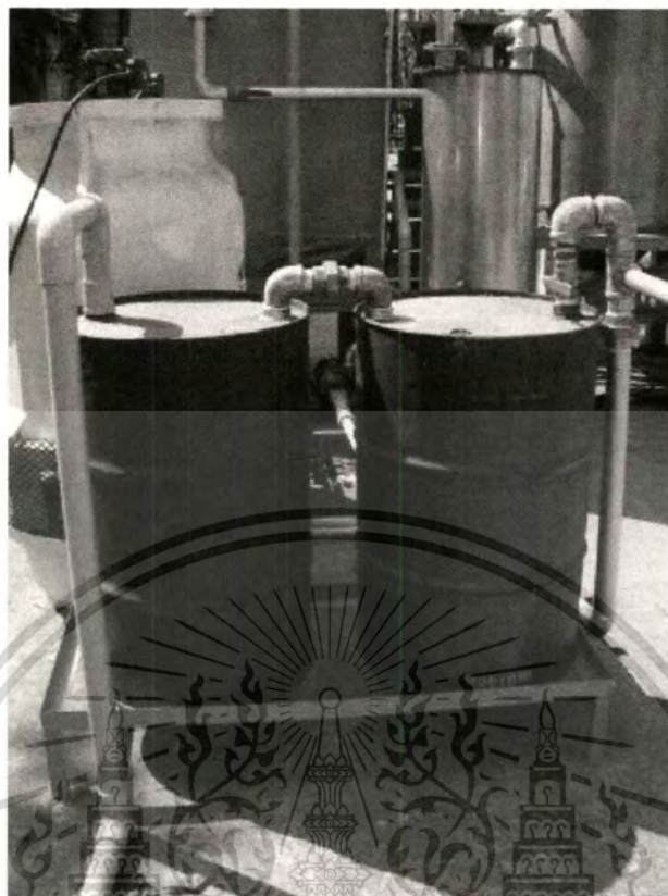
Fig. c.14. The gas tanks.
