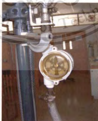
Fig D4. Cooling water is opened automatically when start the process.
