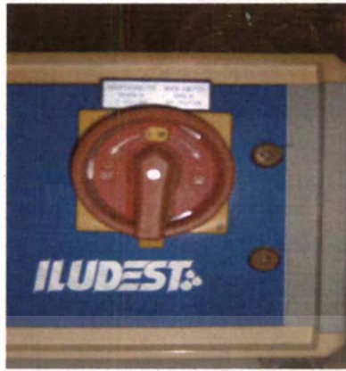
Figure 3-5. Main switch of the distillation tower system
